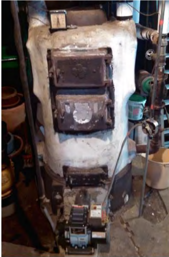
Boiler wrapped in asbestos insulation Picture from Expanded HEAT Loan Initiative Report , December 2015, E4TheFuture.
